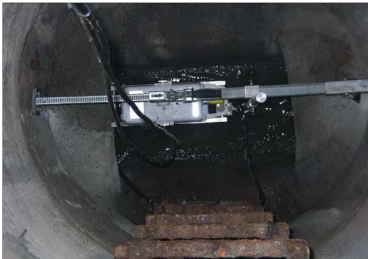
The meters are installed above the flow to minimize maintenance issues and the cost of confined space entry of sending city personnel for meter repairs.
