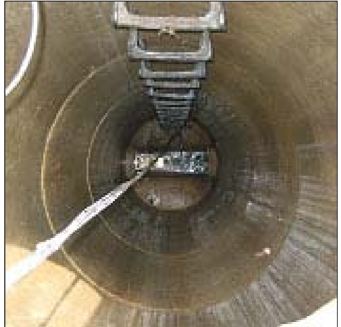
DDS Flo-Dar Sensor installed in 14" Line – Case Road
