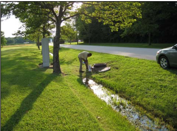
DDS Flo-Logger electronics install – Abbe Road
