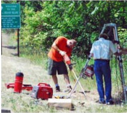
Installing a digital cellular antenna at one of the Data Delivery Services sites.
