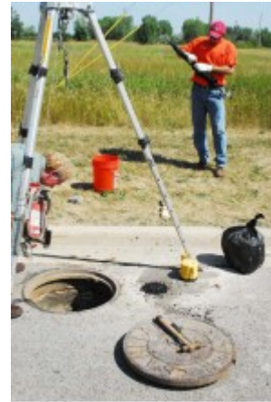
Dave Baker (foreground) assists in the installation of the Data Delivery Services flow metering network.
